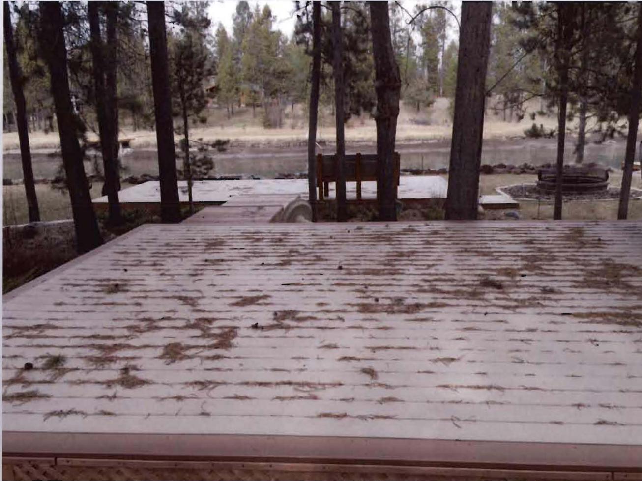
The landscaping decks located on the property, looking north toward the Deschutes River from the south edge of the southern landscaping deck, with the walkway and north landscaping deck visible in the background. Photo taken 2/25/15.
