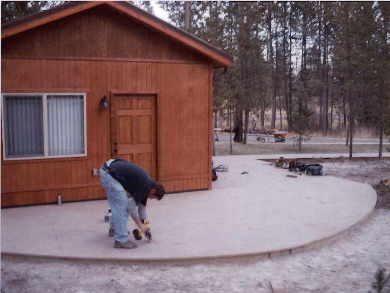
The south side, or backside, of the Bath House, looking northeast during the final stages of construction of the exterior decks. Photo taken Winter of 2009.
