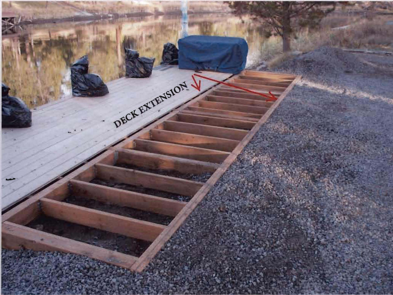
Construction of the over-land platform, which connects to the over-water dock, on the northern edge of the property, along the Deschutes River. Photo taken Winter of 2009.
