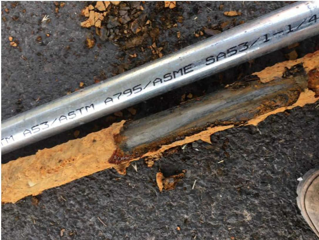
Iron encrustation and staining on the pump column below the water table.
