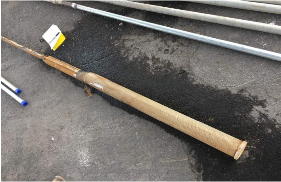
Existing 5 hp submersible pump removed from the well. Note the iron staining and scale on pump.
