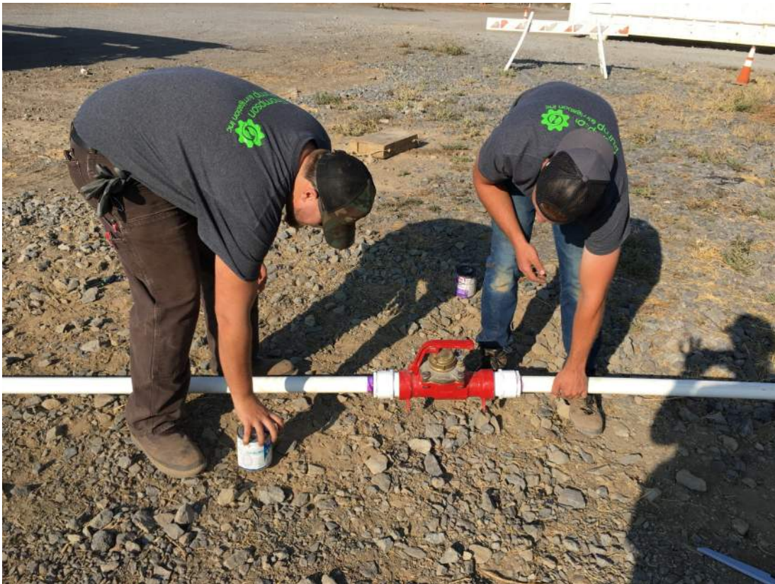
Plumbing of the discharge pipe and flow meter for the pumping tests.
